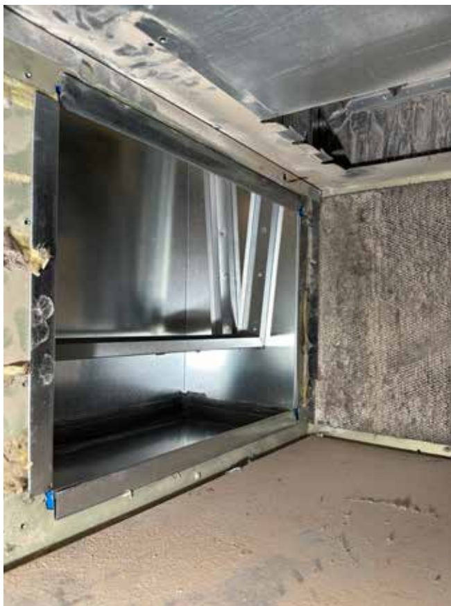
(Furnace blower compartment with blower removed to give photo access.)
